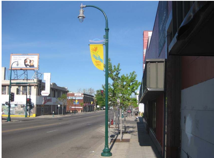
Street Light Pole and Luminaire (Partial enhanced cost) Enhanced Elements - Banner brackets & GFCI circuit
